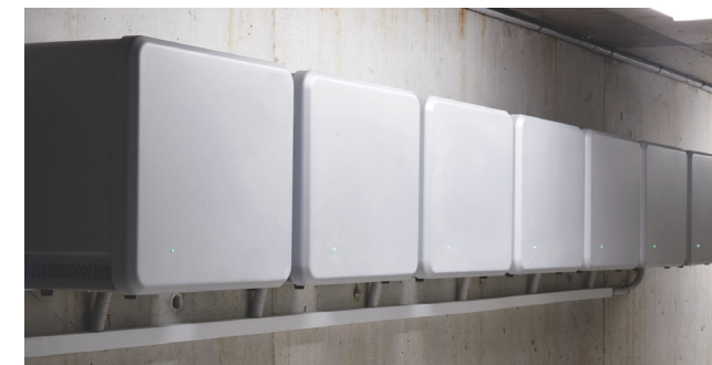
Wall-mounted lithium battery
